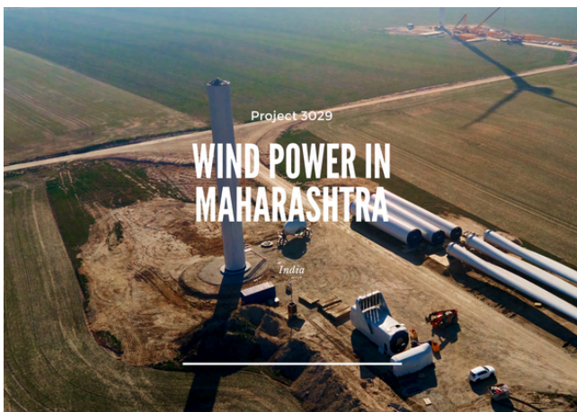
Project 3029: Wind Power in Maharashtra
